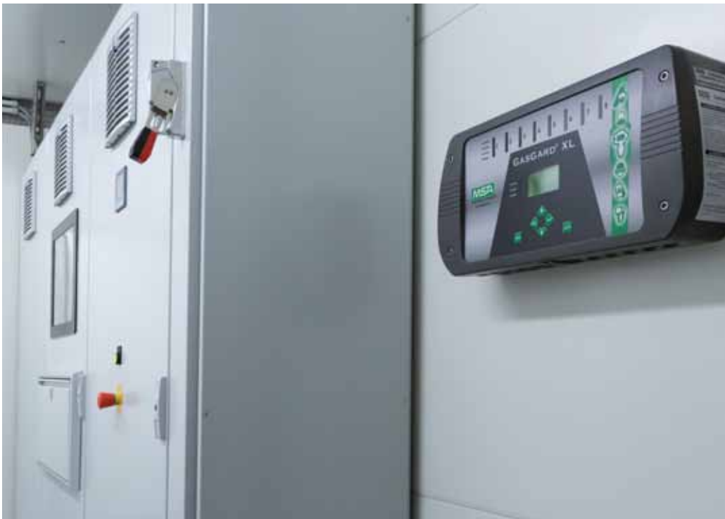
On-site control cabinet inside containerized OilPaq
